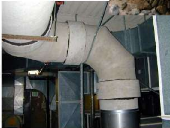
ASBESTOS CEMENT LAB FUME HOOD EXHAUST DUCT
